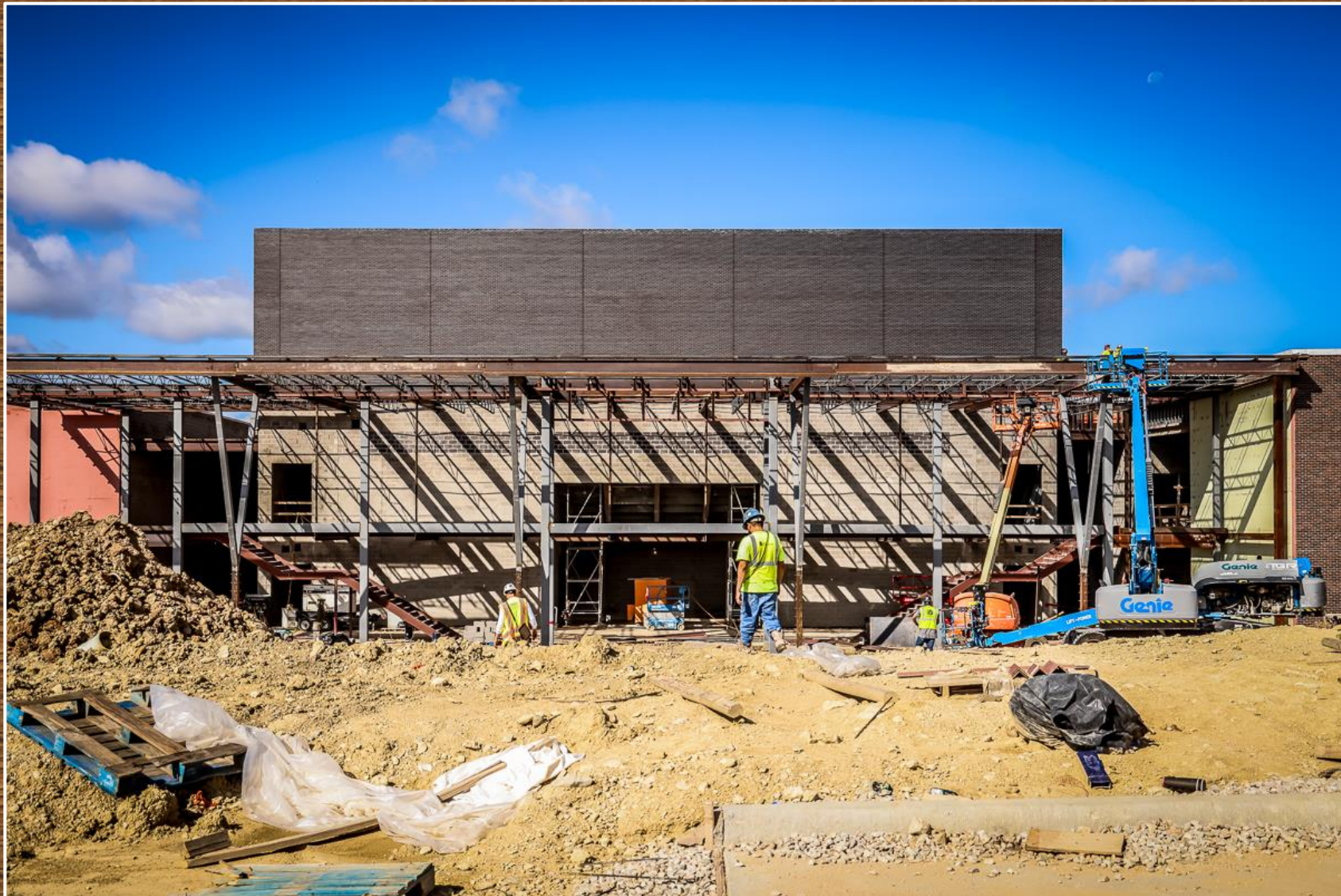
Structural steel installation on the main entrance to the PAC is in progress.
