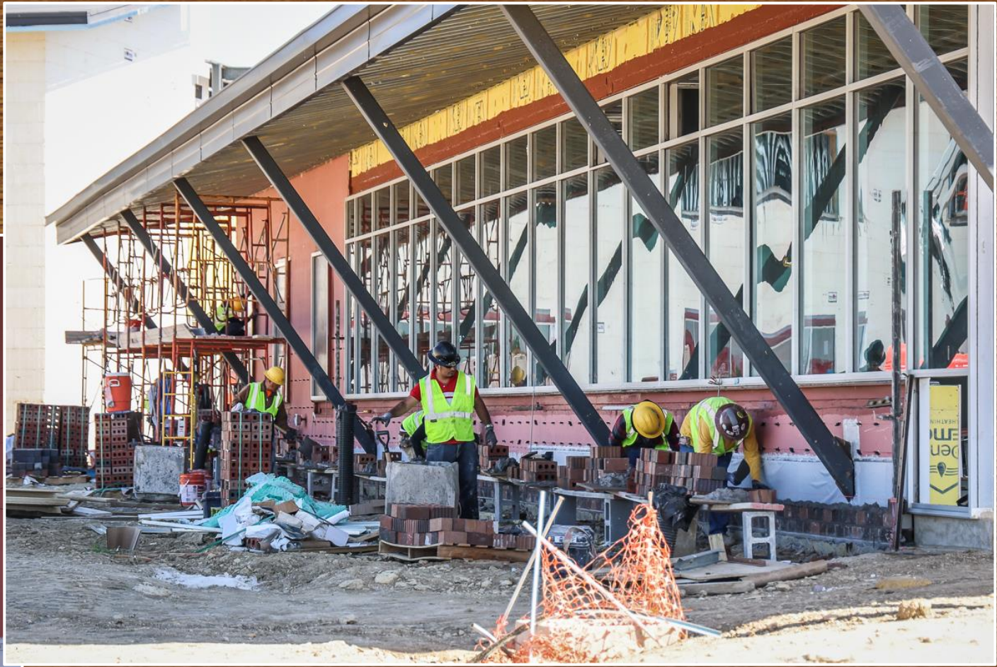
Brick and rock installation are progressing on the administration and library areas.
